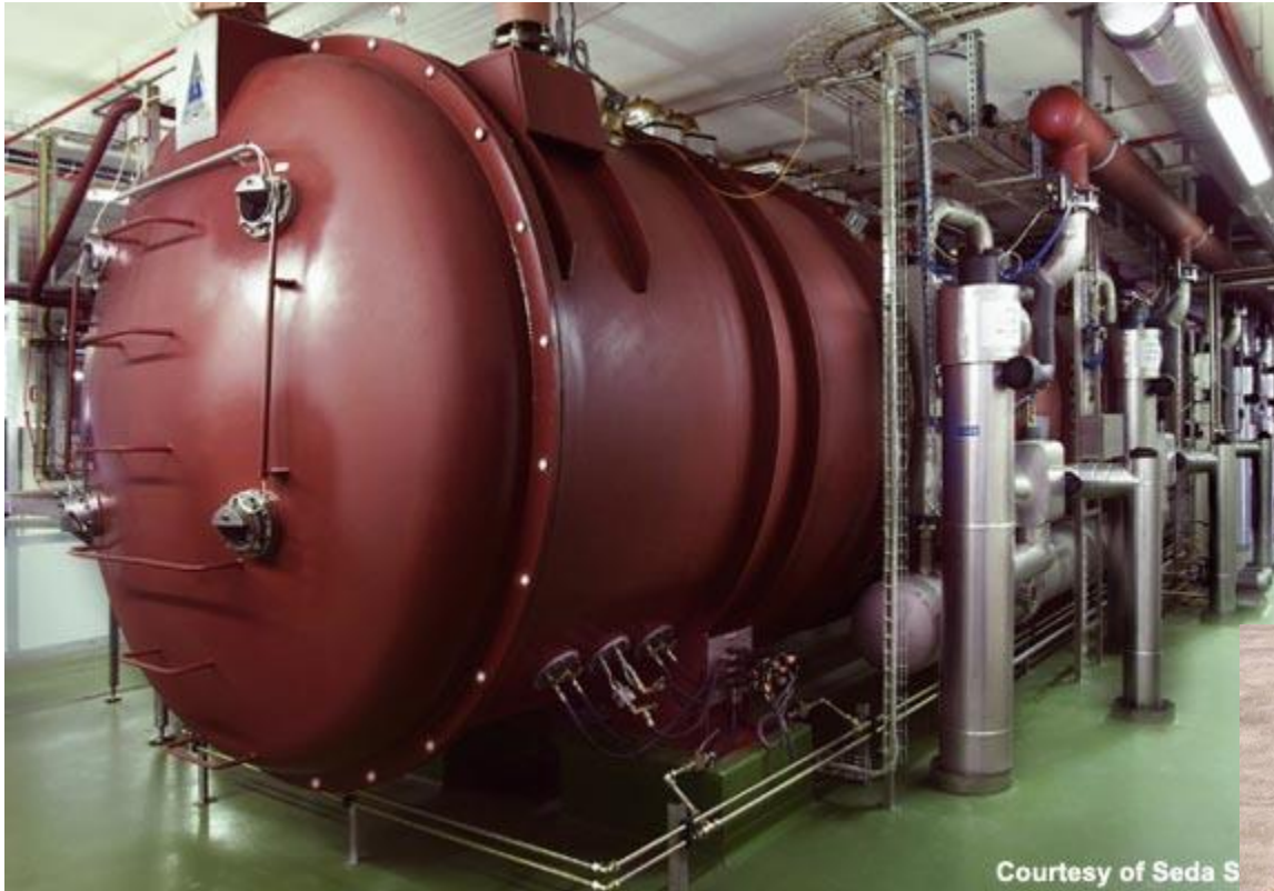
ConRad 500 freeze-drying equipment has been installed at the Seda Solubles facility.
